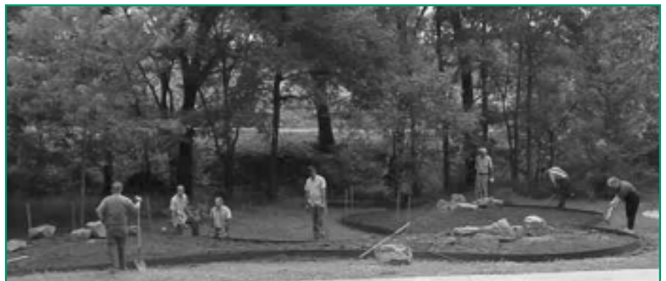
Commission members, Parks & Recreation staff and Master Gardeners break ground on the Xeriscape Garden located on the Greenway near Hollywood Park.
